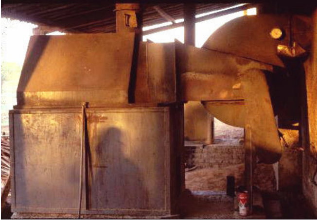
Figure 4. Wood fired heat exchanger on outside of building.
