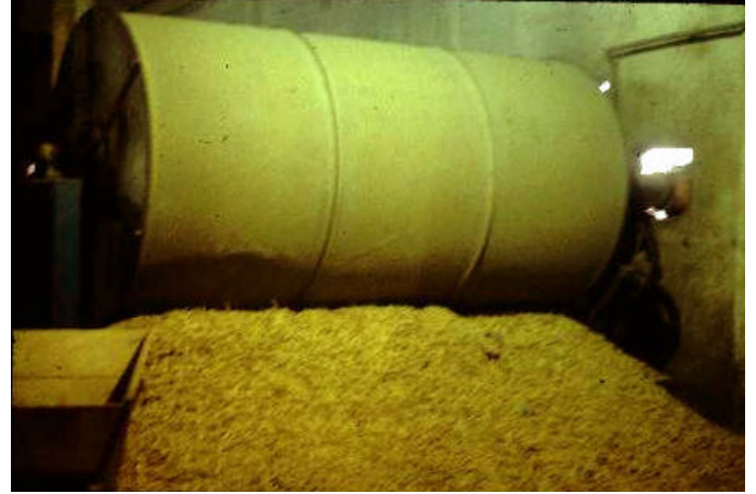
Figure 5. Rotary coffee dryer with heat provided by wood exchanger
