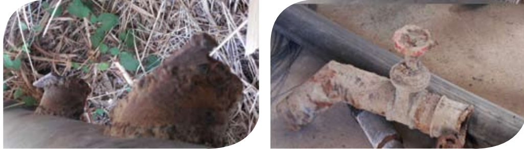
Figure 6: Parts of worn out network and illegal connections identified and isolated by the WUA.
