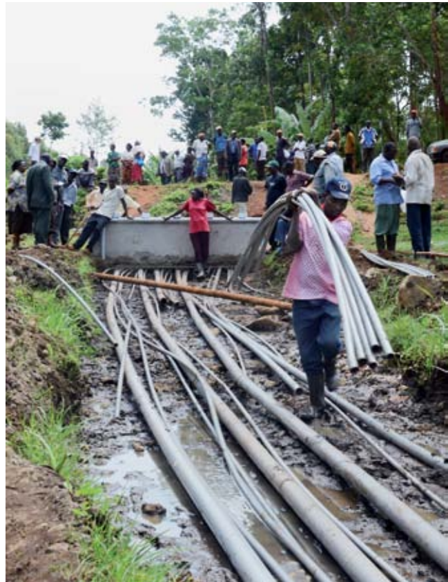
Construction of a common intake (a central place where water is allocated and metered for 17 small scale projects). Meru, Kenya.
