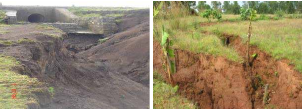
Figure 43. The destructive effects of road drainage upon land in Oromia Regional State - West Harerghe (left) and Ghimbi (right)
