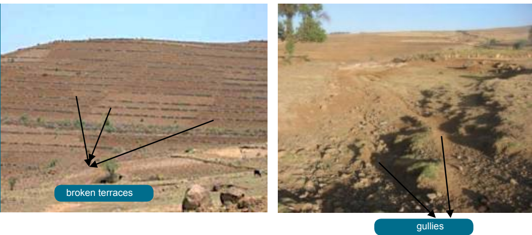
Figure 8. The damaging effects of improperly built, degraded or unmaintained physical structures
