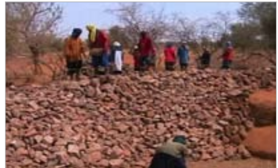
Closing off a gully with a permeable rock dam. Source: PGRNG Mauritanie
